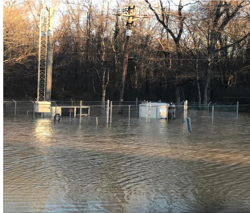
Ellis Road Pump Station
