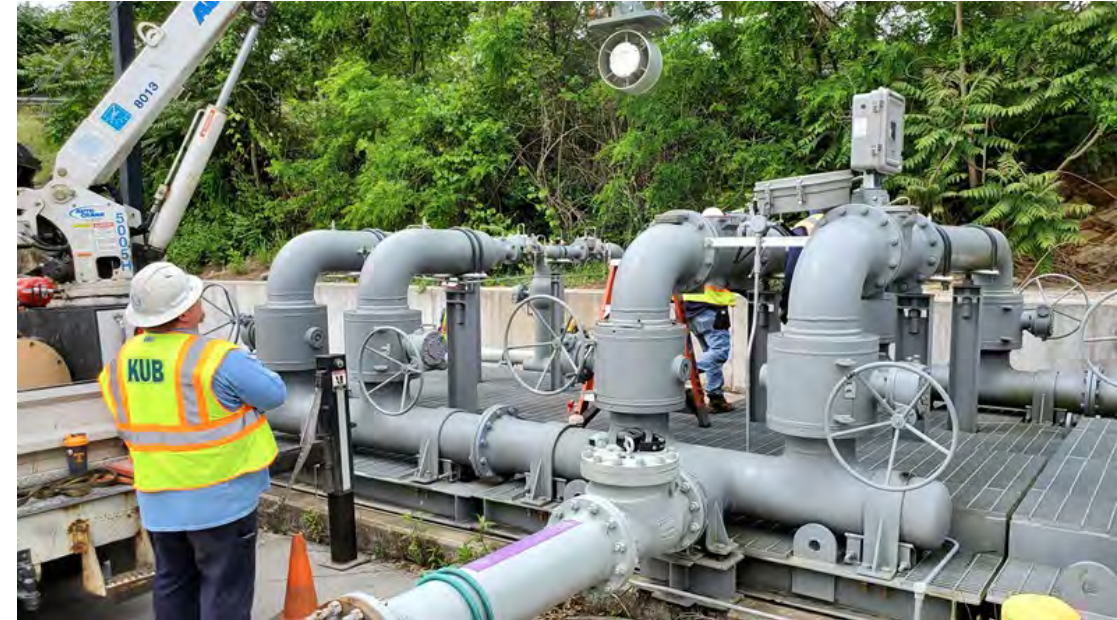
UT Cogen Natural Gas Meter and Regulating Station
