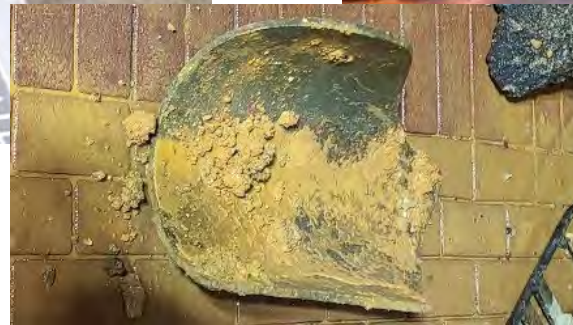
Piece of main removed
